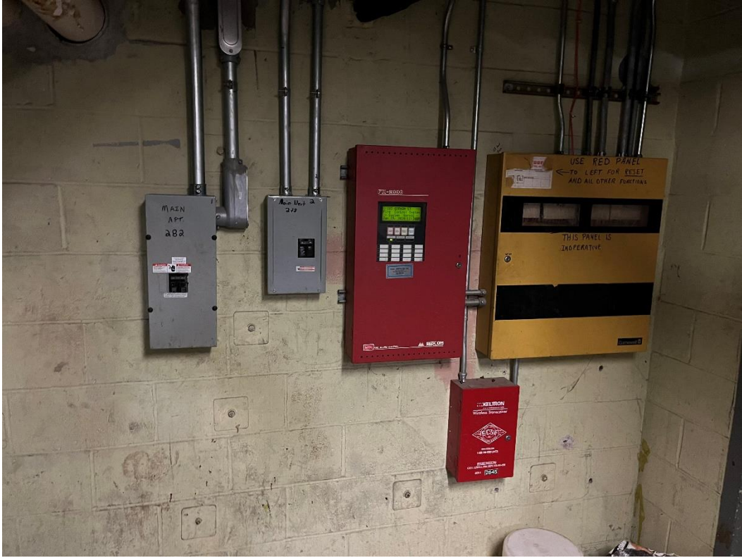
Alarm at 183 Gorham Street
