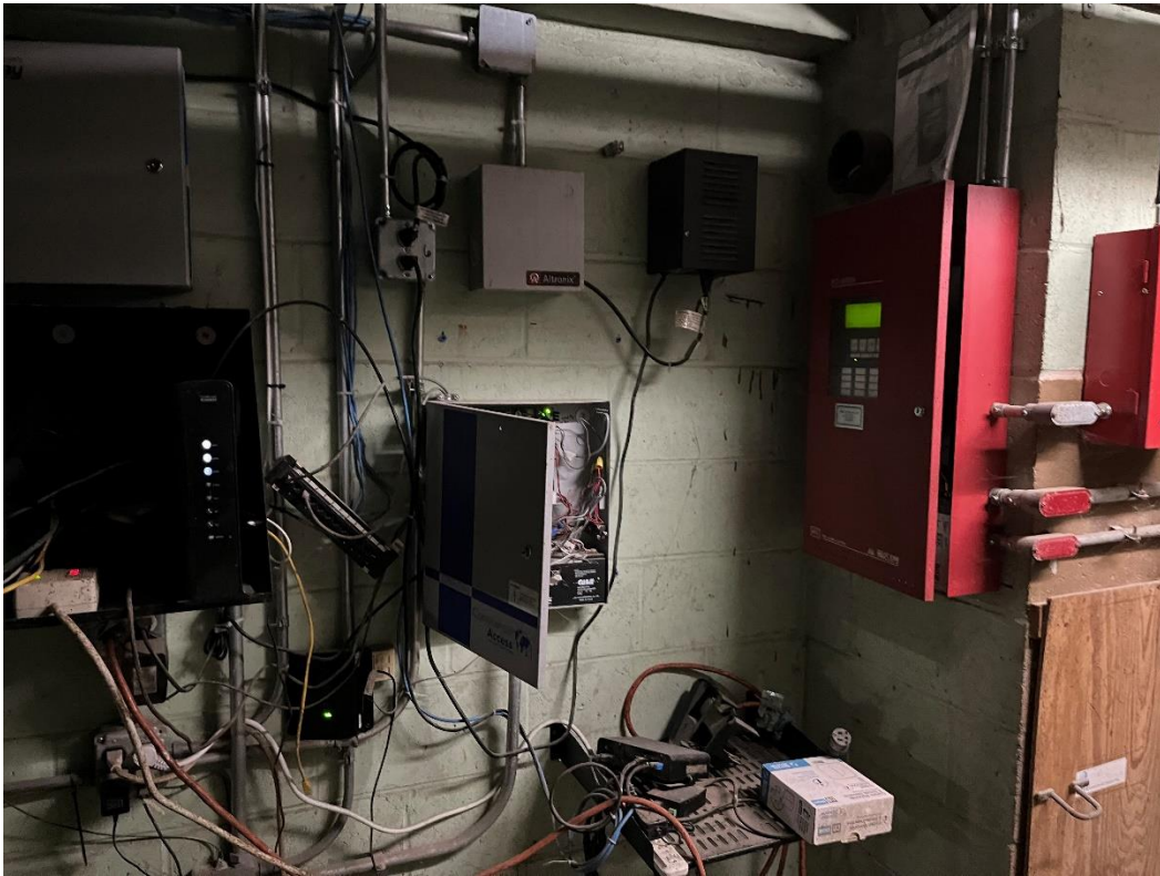
Alarm at 145 Gorham Street
